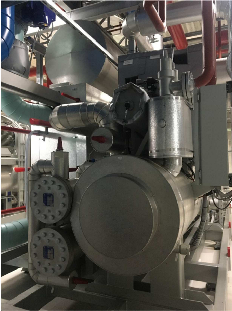
Image 3. One of the new heat pumps that transform datacenter air into district heating.
